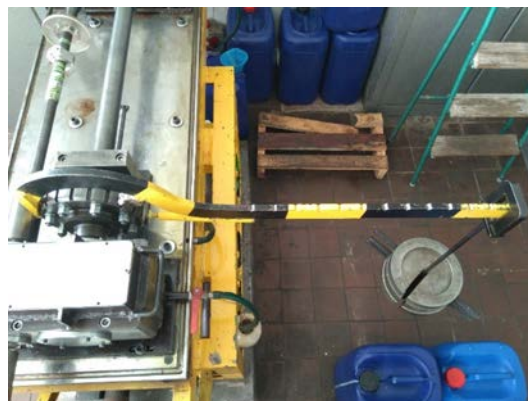
Fig. 3. Three-phase electric motor of Niemann M01
